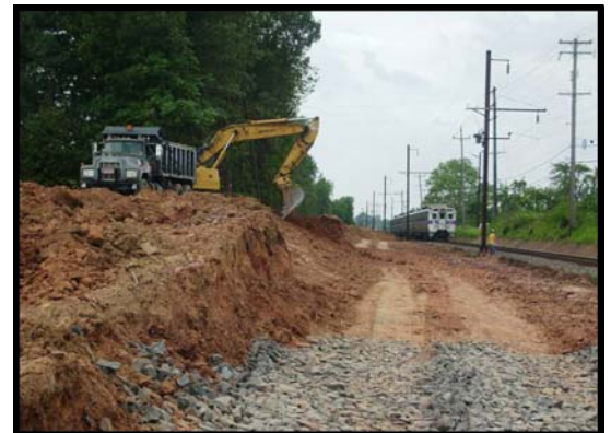
SEPTA: Link Siding; Doylestown, PA Architect: HNTB Corporation
