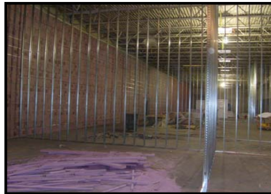
Drummond Road Office Warehouse Philadelphia, PA Architect: AECOM Services of PA, Inc.
